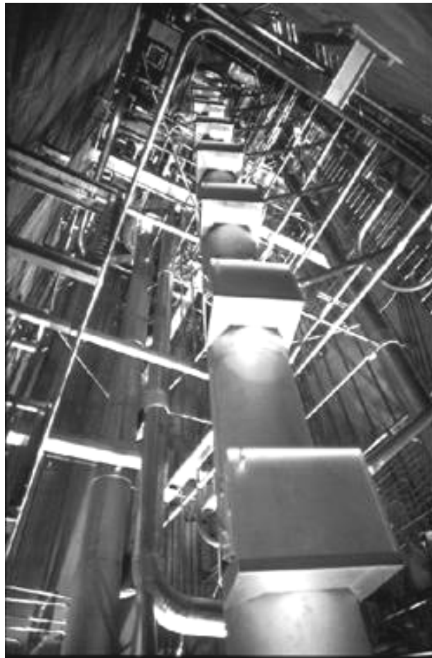
Figure 7.6. Pulsed column in the T2 facility at La Hague (Source: COGEMA – France)
