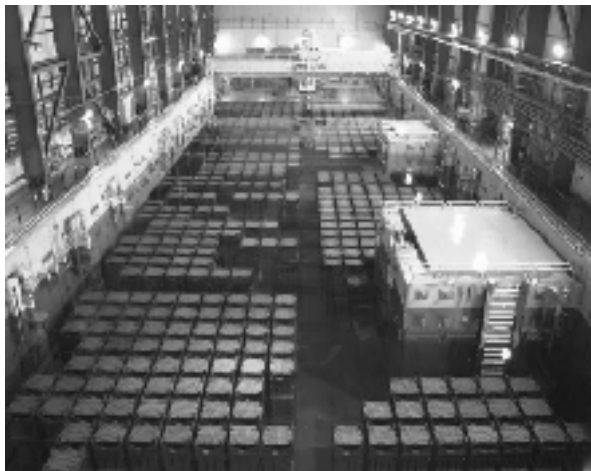
Figure 6.1. Pool storage (Source: COGEMA – France)
