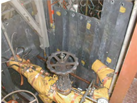
Installation of biological shielding on a pipe enabling monitoring of a valve
