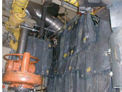
“Bracelet” type protection on a pipe
