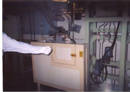
Fixed biological shielding with an access hatch for checking a valve at Almaraz NPP
