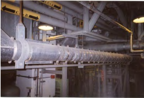
Permanent lead shielding on a pipe in the Almaraz nuclear auxiliaries building
