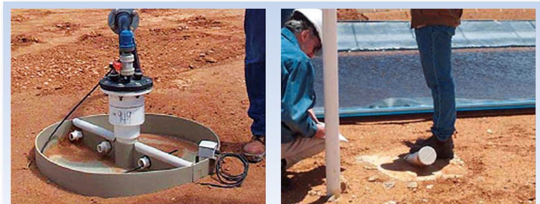
Wellhead with drip tray and online detector (left); evaporation pond with leak monitoring (right) at the Beverley ISL mine. A comprehensive environmental impact assessment (EIA) process based on a thorough understanding of local site conditions, field trials and baseline environmental data that demonstrated well field containment was required before approval to begin operations. Ongoing environmental monitoring provides assurance that the facility is operating as planned.
