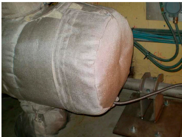
FIG. 3. Improper insulation installation.
