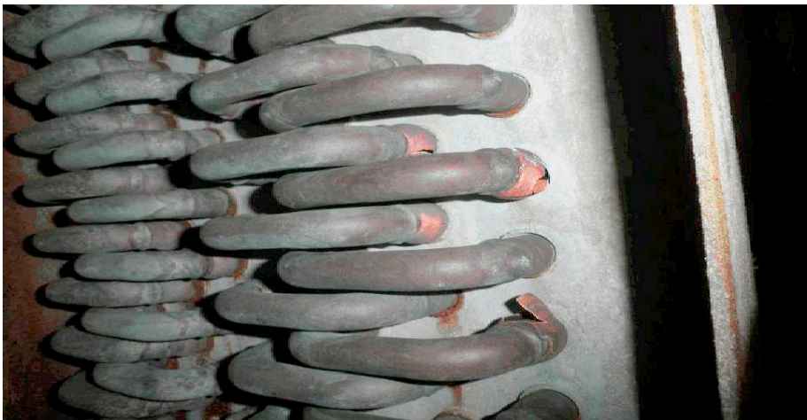
FIG. 7. Heat exchanger tubes, showing origin of leak.
