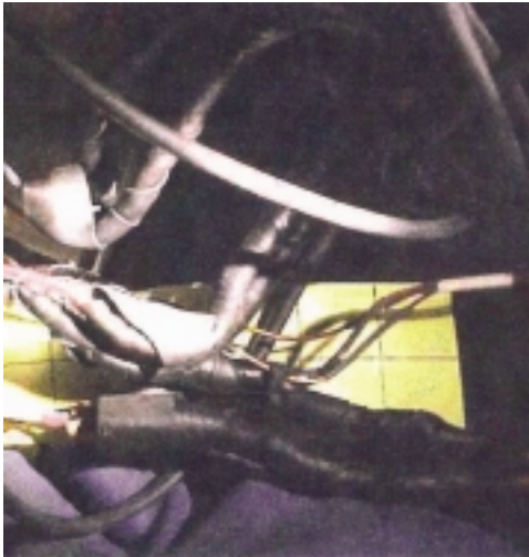
Environmental ageing of components such as electrical cables is of importance in maintaining safety of associated components and systems (source: USNRC).
