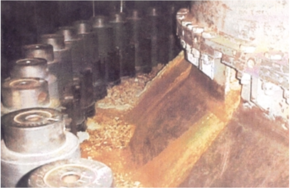
This photograph shows the effects of buildup and concentration of boric acid near the bolting area where the upper head attaches to the main portion of the reactor vessel (source: USNRC).
