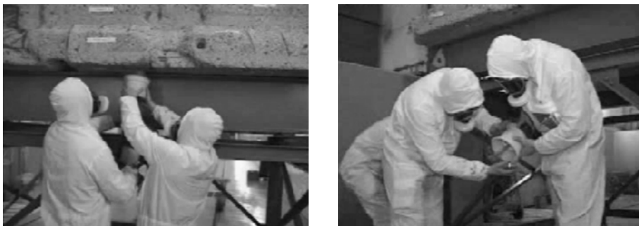
Figure 4.1 Taking samples at concrete surfaces with a power drill with milling head and a beaker to collect the powder (left); transferring the powder to a measurement container (right) (pictures from [KWW, 2004])
