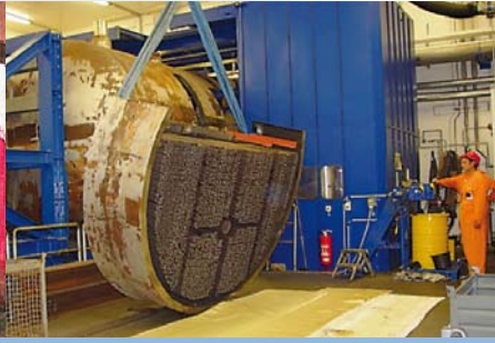
Cutting of a steam generator with a large band saw in the Interim Storage Facility North (ZLN).
