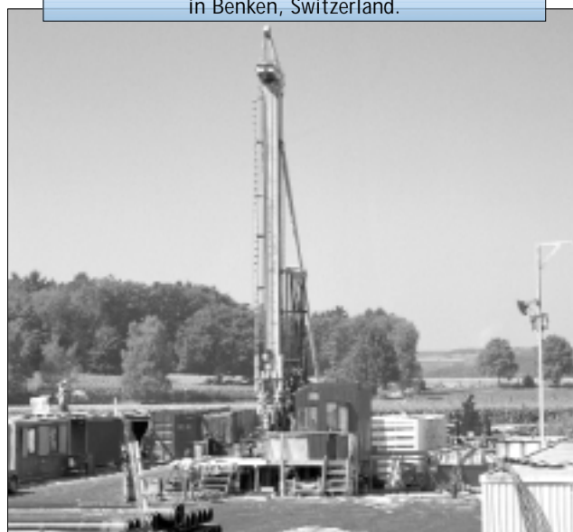
Geological and hydrogeological exploration of a mesozoic clay formation (opalinus clay) in Benken, Switzerland.
