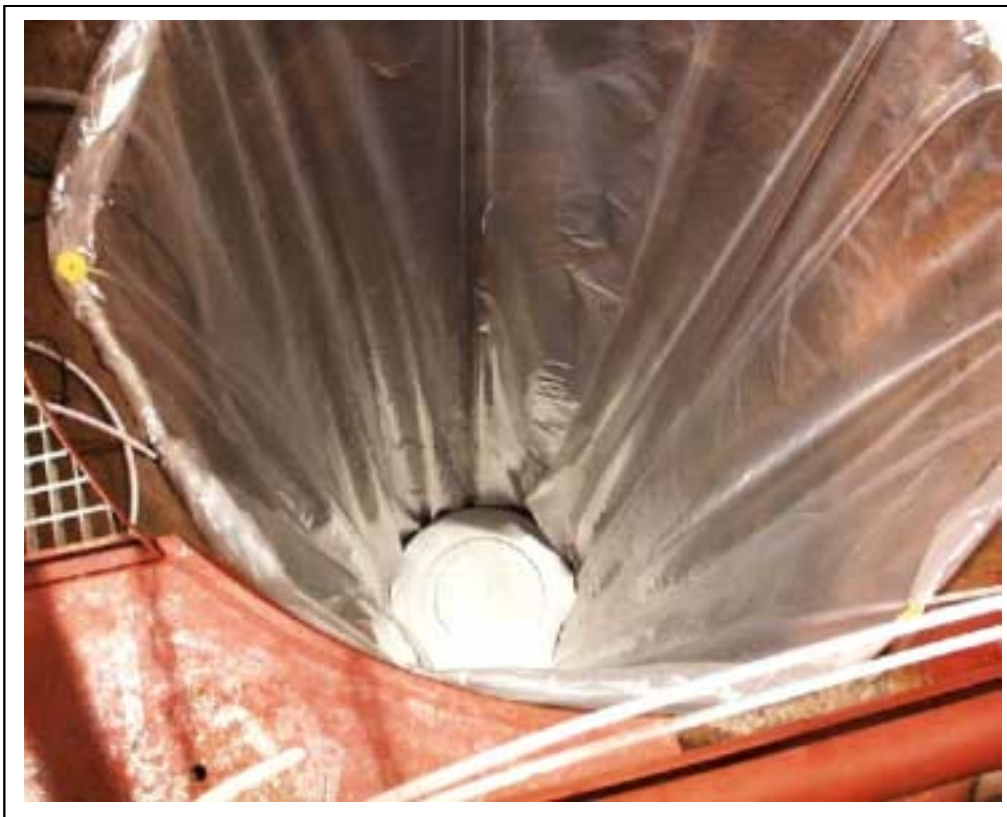
Figure 3.7. A Spent Fuel Deposition Hole Lined with Plastic to Control Water Inflow (The disc-shaped object at the base of the hole would form the bottom of the bentonite buffer)
