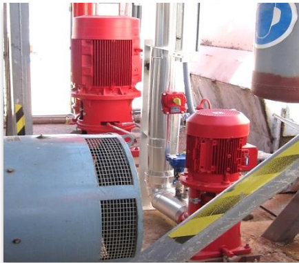
New fire protection pumps.
