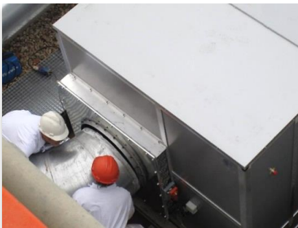
Ventilation system adaptation.
