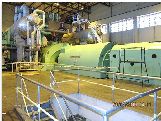
Initial status of the operational plant.
