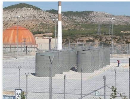
Independent spent fuel storage installation.
