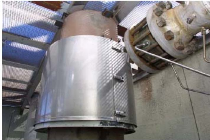
Figure 2-7: Outside View of the Collection Chamber.
