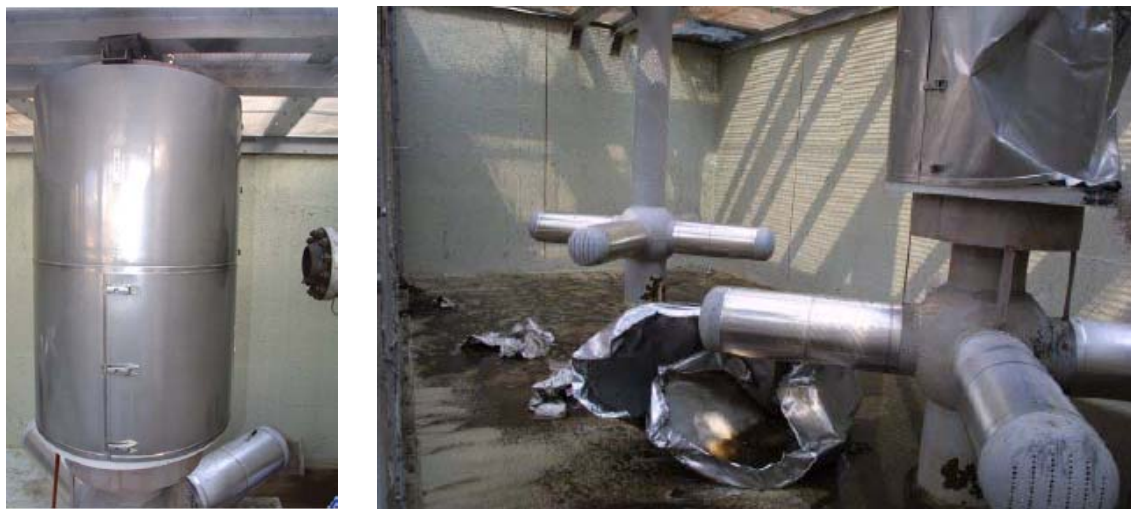
Figure 2-12: Left: Position of lower cassettes with one in front of the jet and one away from the jet and upper cassettes with the interface in front of the gap, jet outlet at the right side Right: Removed and destroyed upper cassettes at the floor and deformed lower cassette faced to the jet, jet outlet out of the picture bottom right [2-43].
