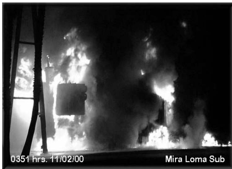
Fig. 3.10-3 Fire and smoke produced during a substation fire
