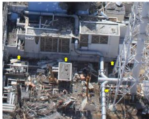
Common ventilation stack of RB3 and RB4
