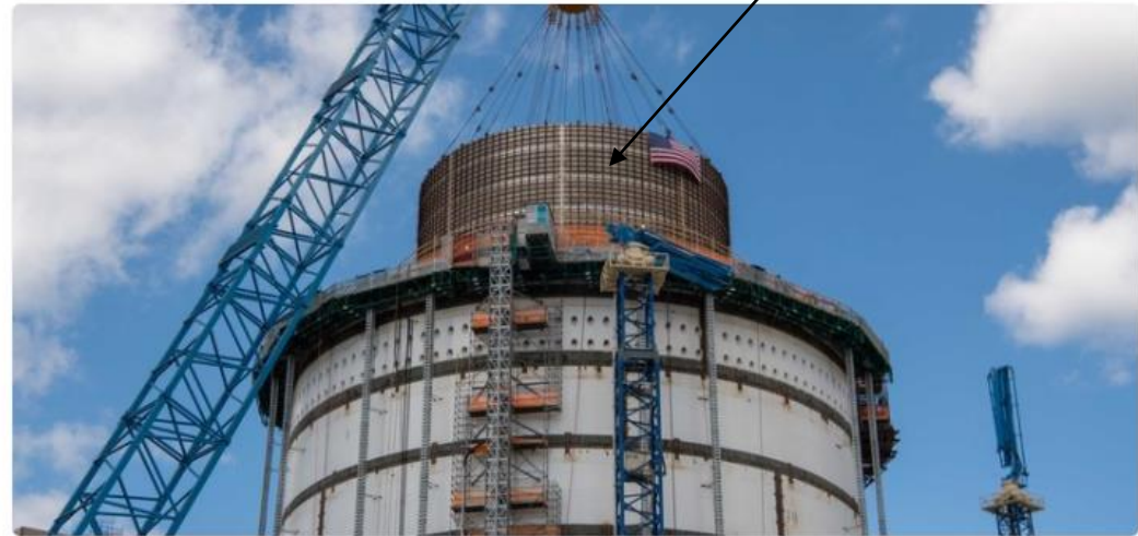
Final Module Installed May 2021 Unit 4 CB20 Tank Holding 750,000 Gallons of Cooling Water
